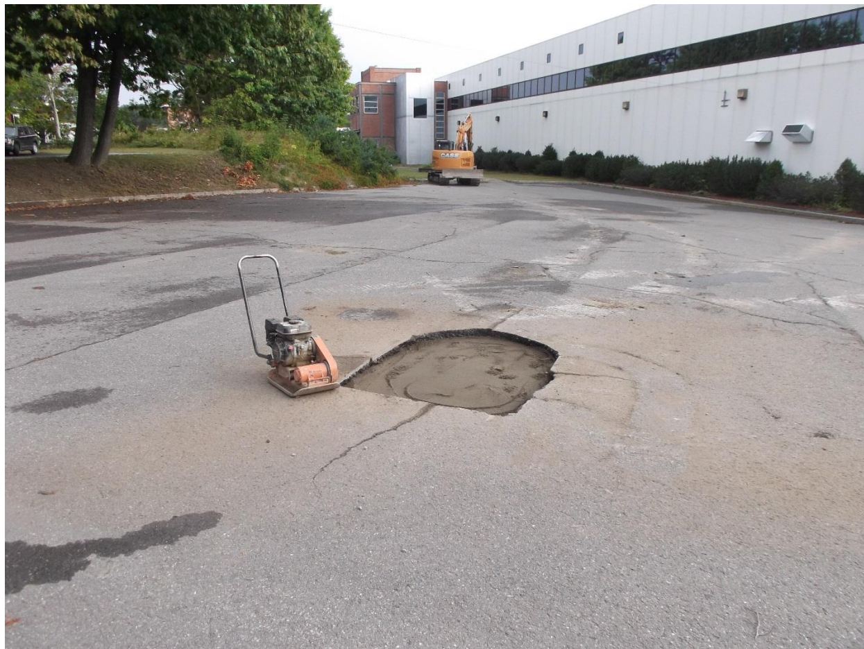
Photograph 1: Conditions following the backfilling and closure of the fieldstone-lined overburden dug well on September 9, 2016.
